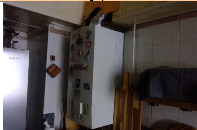
Chaudière type B cuisine
